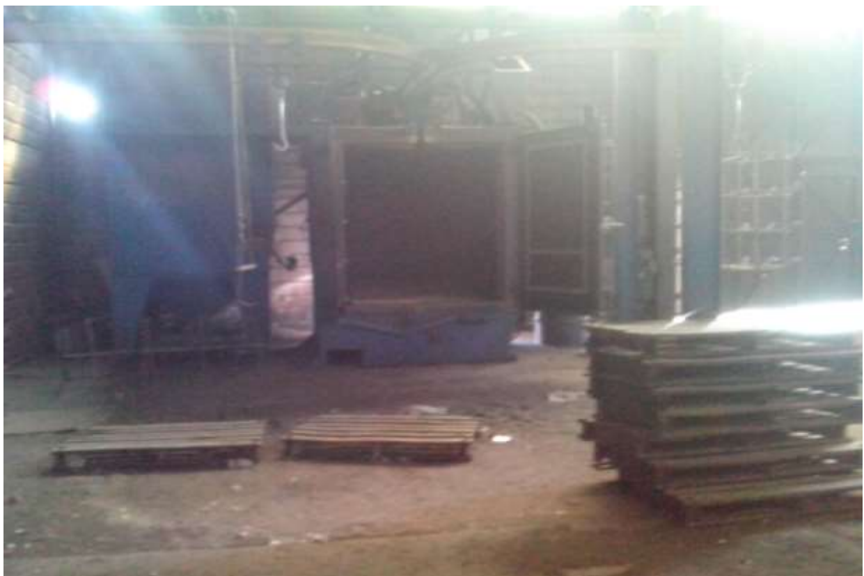
Picture 12 Casting Induction Furnace
